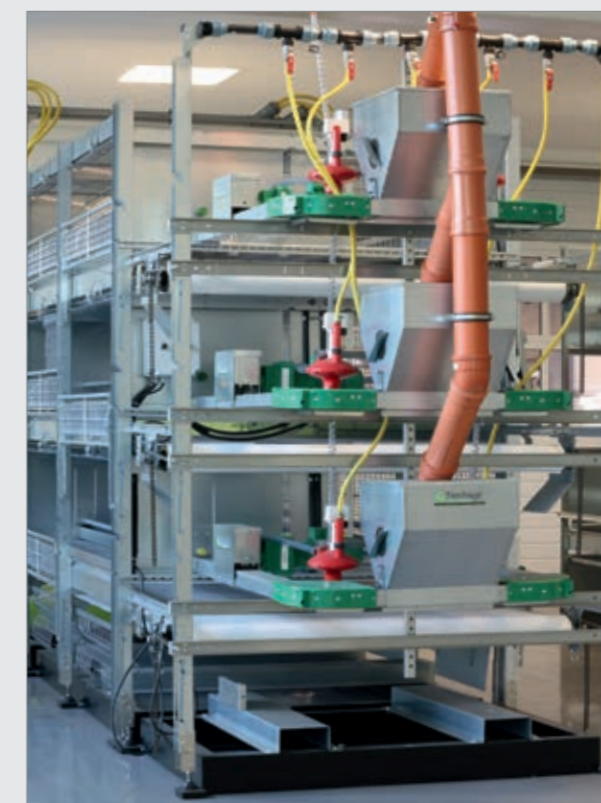
Supply installation in an aviary system
